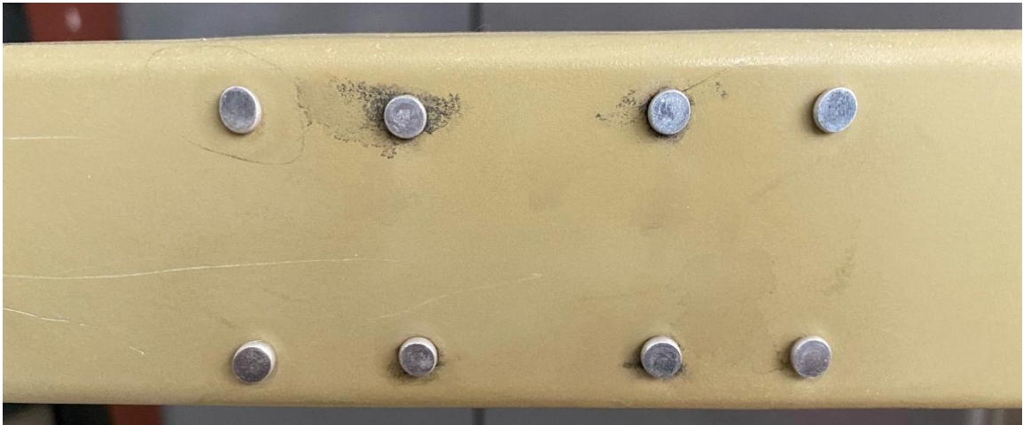
FIGURE 3: EXAMPLE 2 - CRACK LOCATIONS - FWD SIDE OF SPAR
