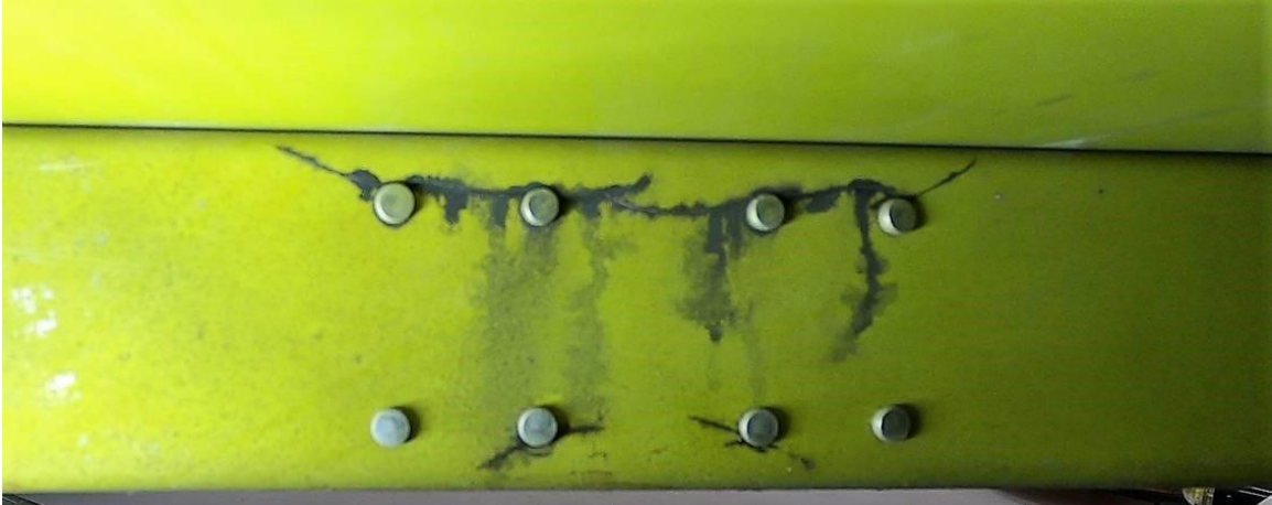
FIGURE 2: EXAMPLE 1 - CRACK LOCATIONS - FWD SIDE OF SPAR
