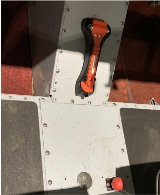
FIGURE 7-11 EXAMPLE EGRESS HAMMER INSTALLTIONS
