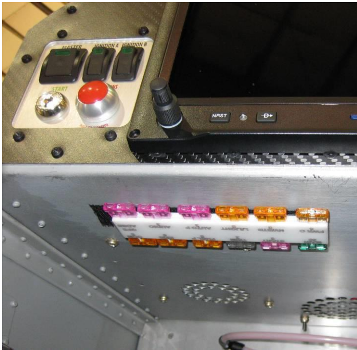
FUSE HOLDER UNDER PANEL
