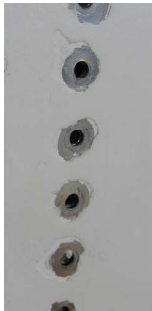
FIGURE 3: REMOVED RIVET HEAD PAINT BUILDUP
